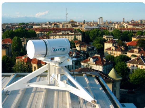
Installation at ARPA Piemonte, City of Torino
